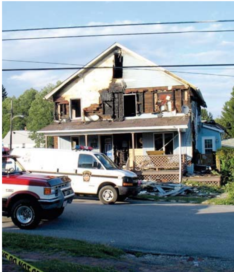
PSP-DuBois are seeking the resident of this house, which was severely damaged in an early-Thursday morning fire in Sykesville. (Photo by Larry McGuire)
